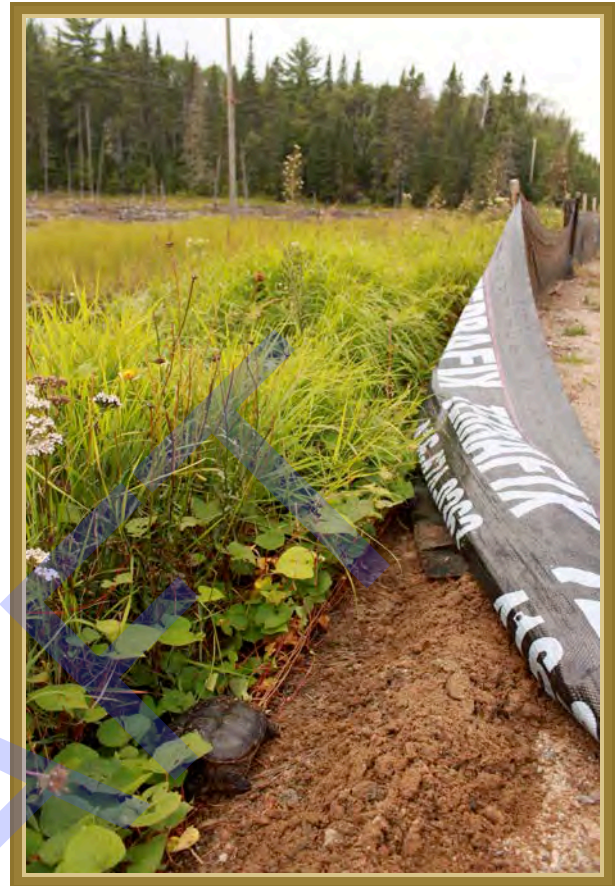
Plate 1. Light-duty geotextile fencing with pre-attached wooden stakes used to exclude turtles from a road as seen on a regular maintenance check (photo credit: Brad Steinberg).
