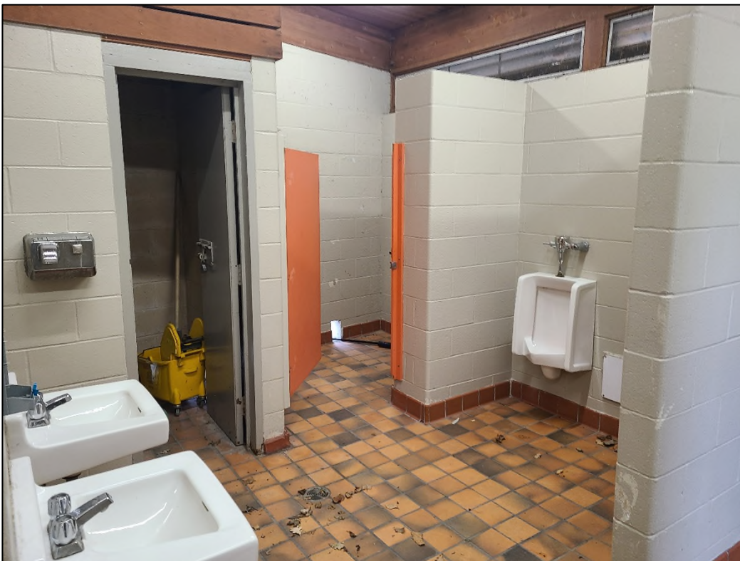
PHOTO 6: WASHROOM IN MAIN BUILDING
