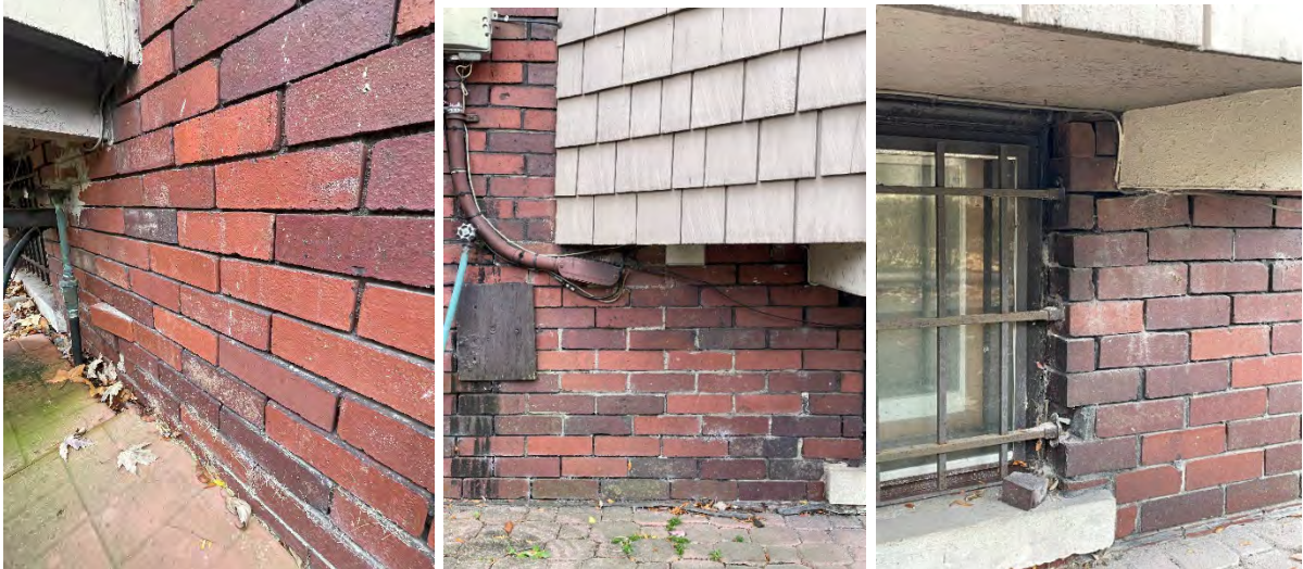
Close-up views of the foundation-level red bricks, showing mortar gaps and loose brick units
