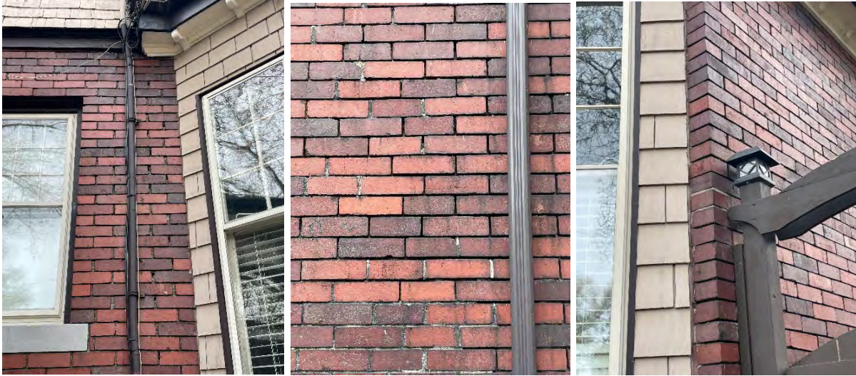
Close-up views of the gaps in the mortar and modern mortar fills on the red brick exterior walls
