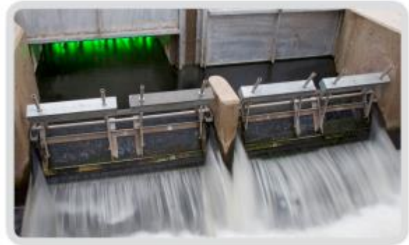
Automatic Level Controller (ALC)
