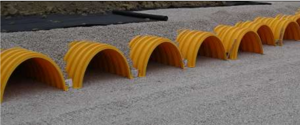
Underground Stormwater Detention System
