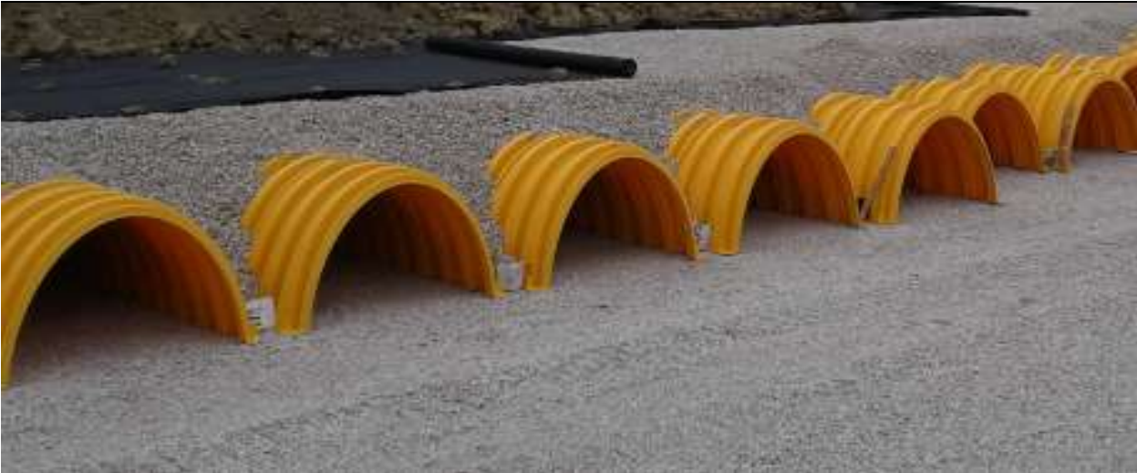
Underground Stormwater Detention System
