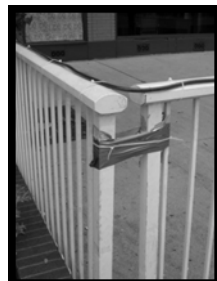
General lack of maintenance
