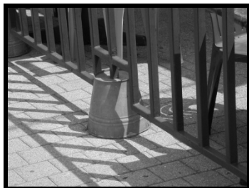
Inverted buckets are not an acceptable means of anchorage/ connection to the sidewalk.
