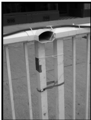
Duct tape and cable ties are unacceptable means of repair.
