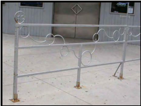
Poor lag-bolt post connections (trip – hazard base bracket)
