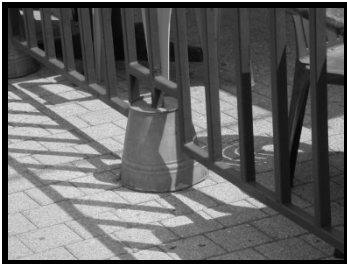
Inverted buckets are not an acceptable means of anchorage/ connection to the sidewalk.
