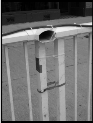
Duct tape and cable ties are unacceptable means of repair.
