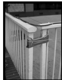
General lack of maintenance
