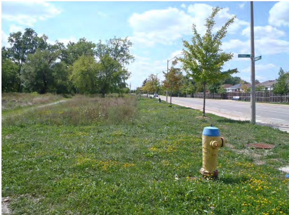
Plate B6: Site conditions showing hydrant line and electrical chamber access cover; looking west
