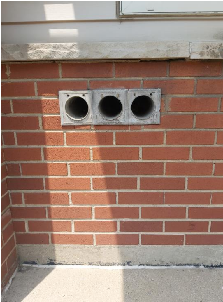
13. Missing / defective grilles.
