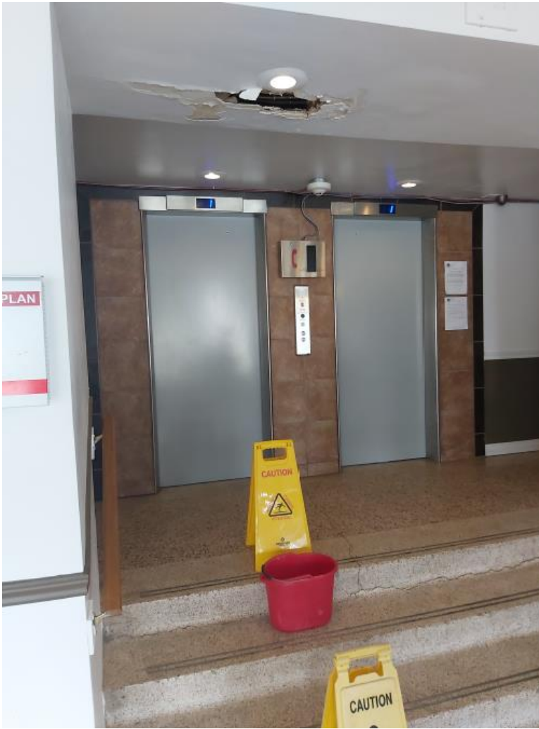
1. Water infiltration in lobby.
