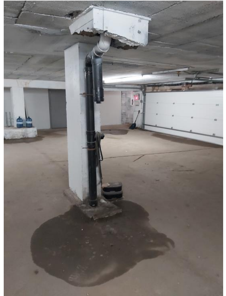
6. Water infiltration in underground parking garage.
