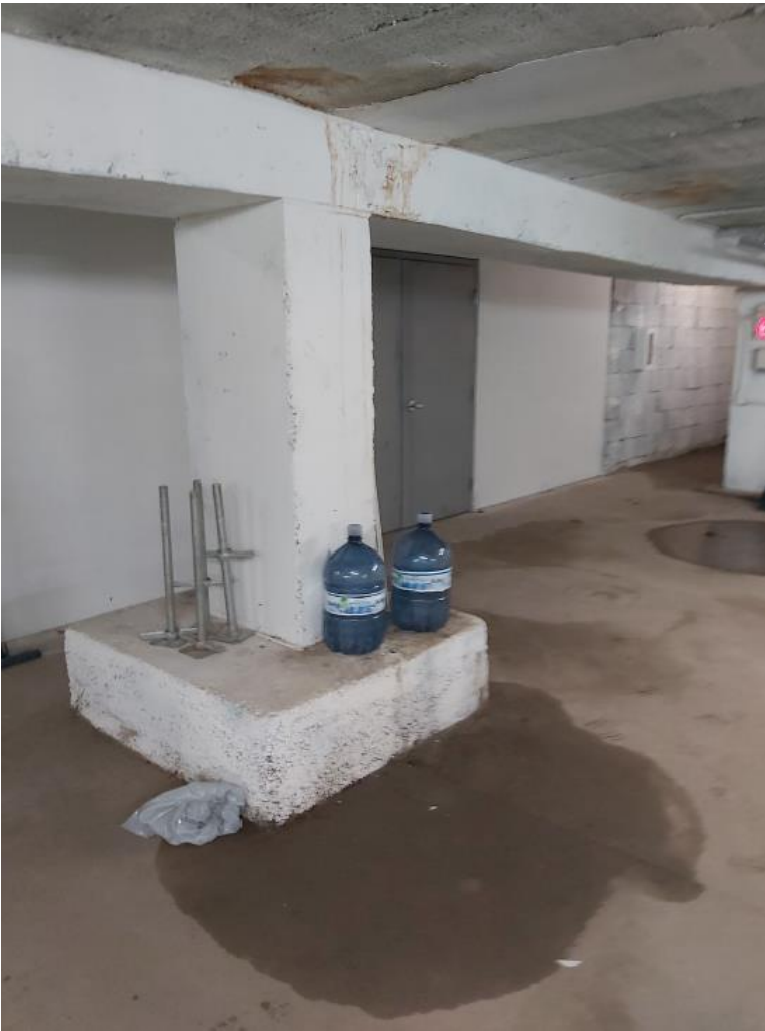
5. Water infiltration in underground parking garage.
