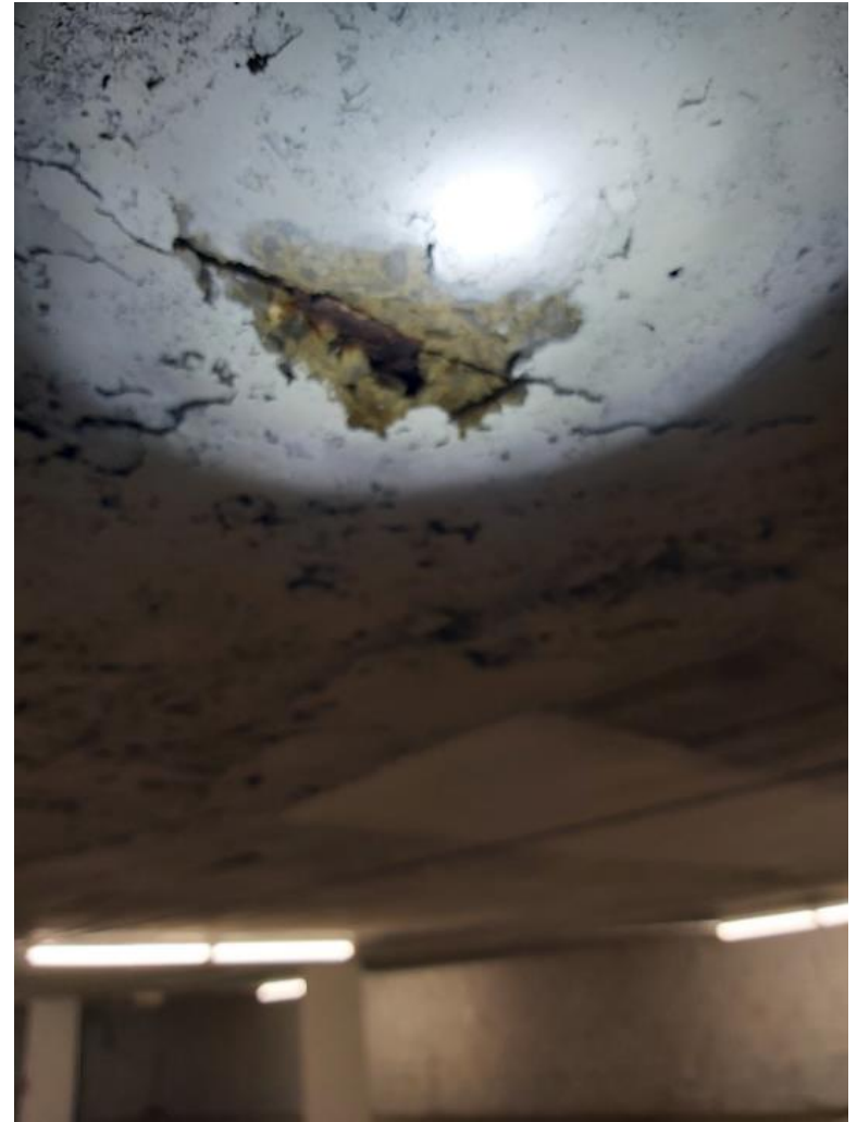
8. Close up of affected concrete structure.
