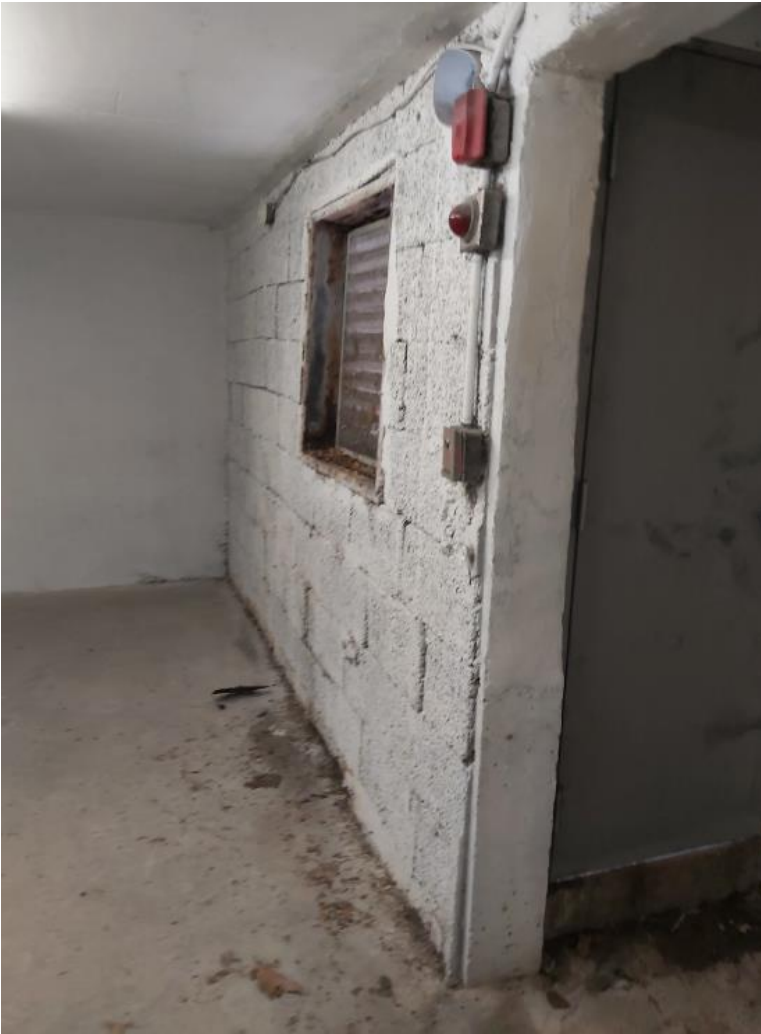
9. Defective exhaust system and defective door from interior.
