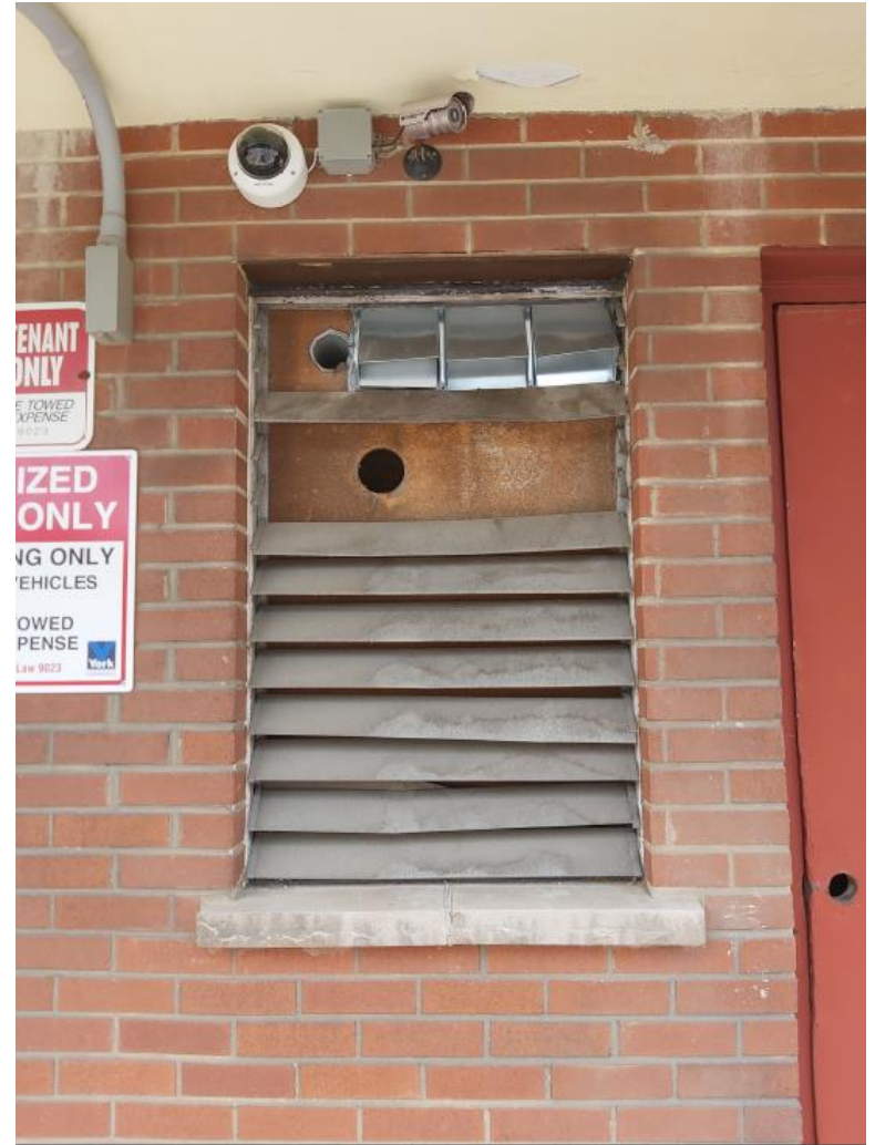
14. Missing / defective grilles. Defective boarding material and defective door.
