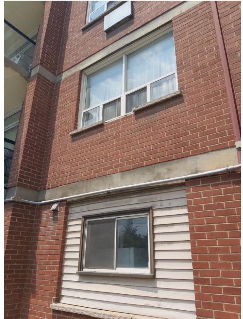
12. Missing concrete window sill.
