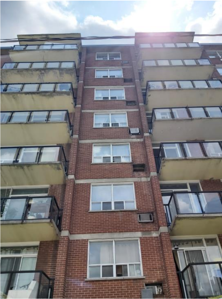
15. Defective balcony slabs and missing air conditioner sleeve cap panels.
