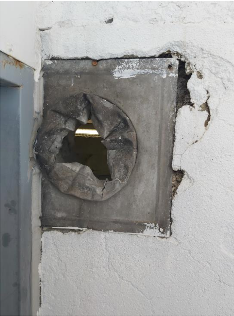
11. Defective exhaust system.
