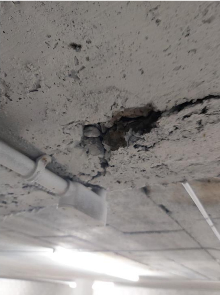
7. Close up of affected concrete structure.
