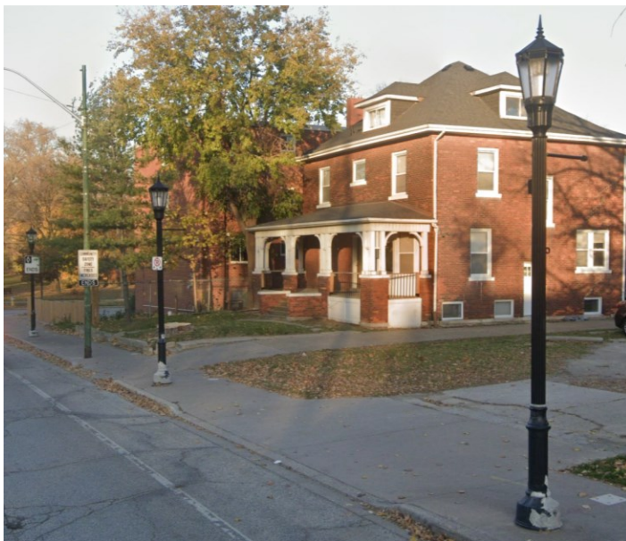
Example of existing black coated decorative light poles where paint has peeled away due to salt damage
