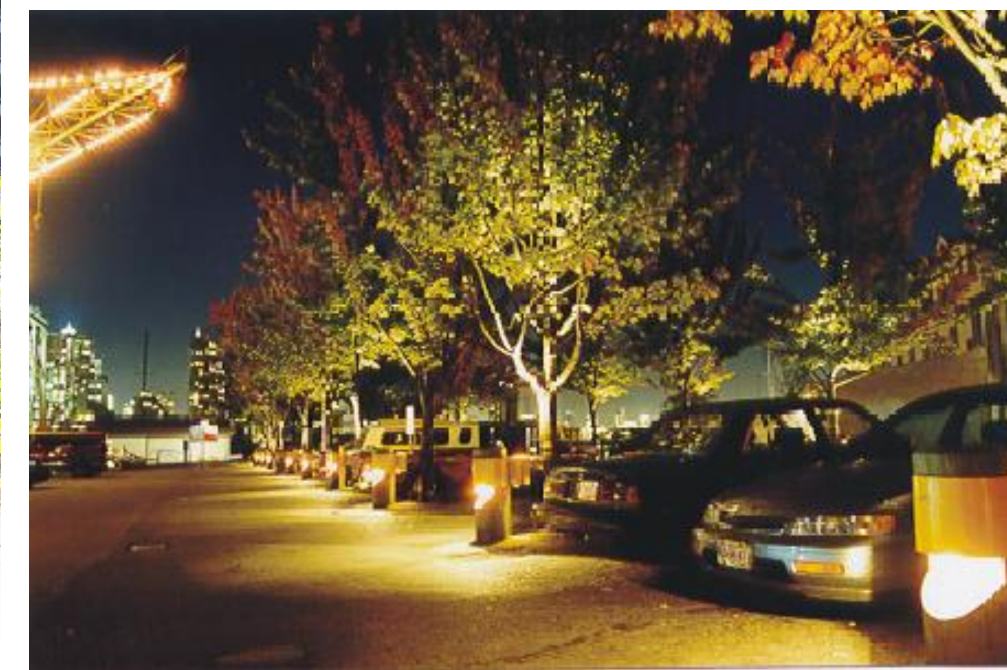
PARKING LOT BOLLARD LIGHTING
